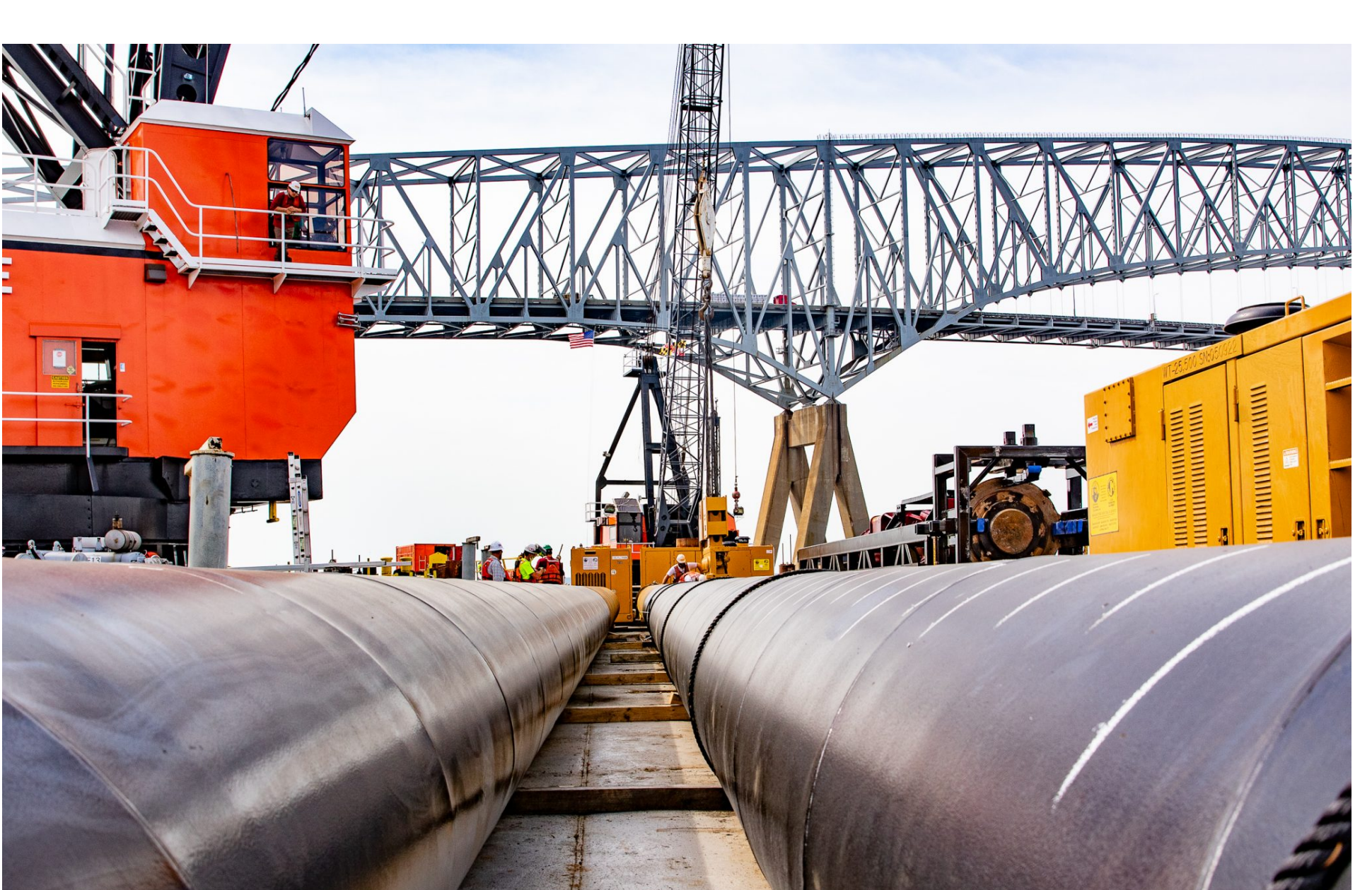
Steel piles await a lift from cranes operated by Glen Burnie-based McLean Contracting.
