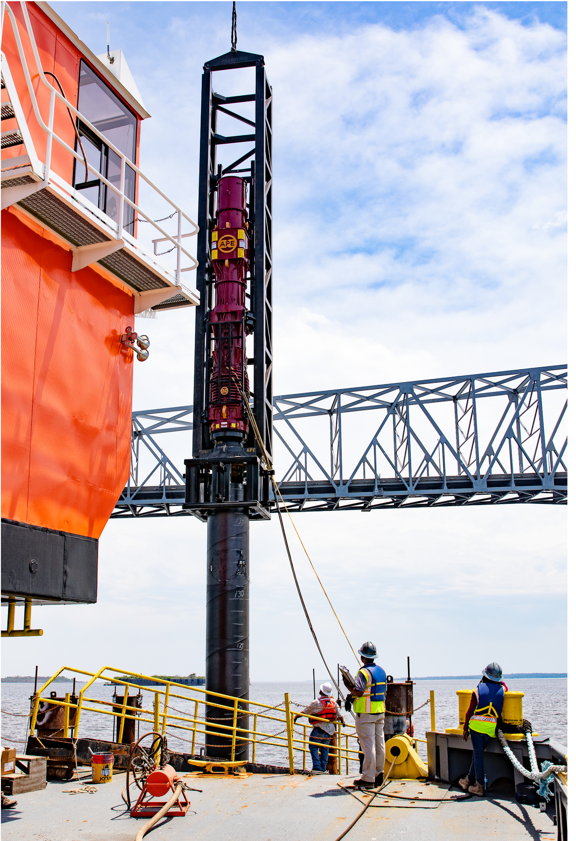
Engineers (foreground) monitor sensor readings while McLean Contracting crews use a diesel impact hammer to complete installation of Key Crossing's first steel pile.
