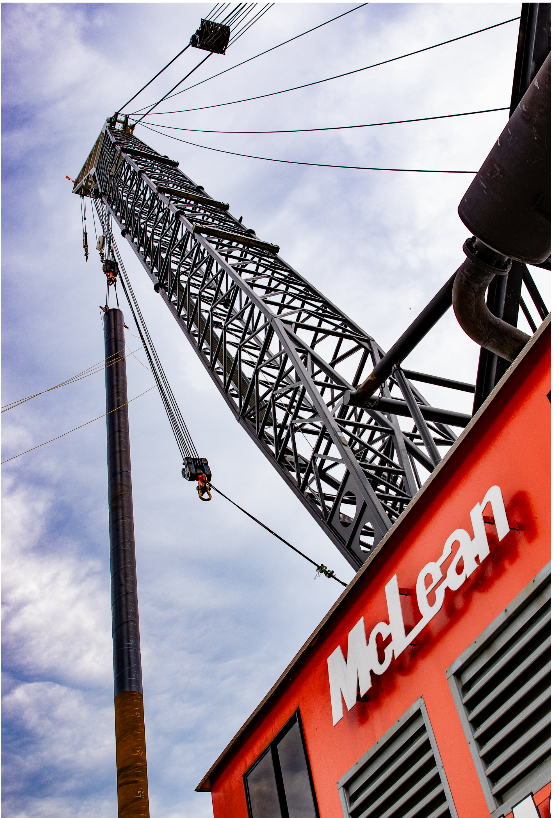
The first Key Crossing Reliability Initiative pile is moved from staging barge to install location in the Patapsco River on June 3, 2020. The pile is one of more than 100 that will be installed this year to support five transmission tower foundations and two vessel collision rings.
