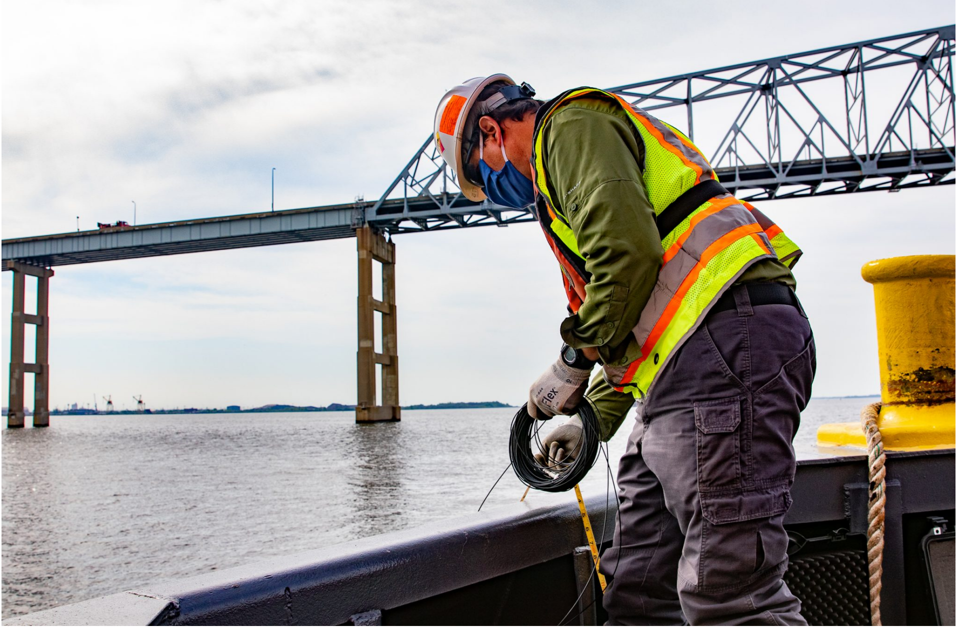
Don Nazario, a senior scientist with environmental consults Normandeau Associates, prepares to monitor underwater sound caused by pile installation work to ensure it stays below levels that could harm fish.
